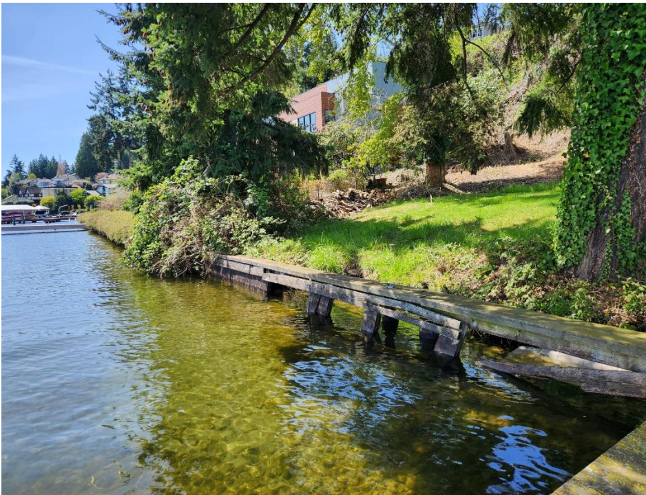
Photo 3. Damaged timber bulkhead and southern shoreline conditions, facing south.
